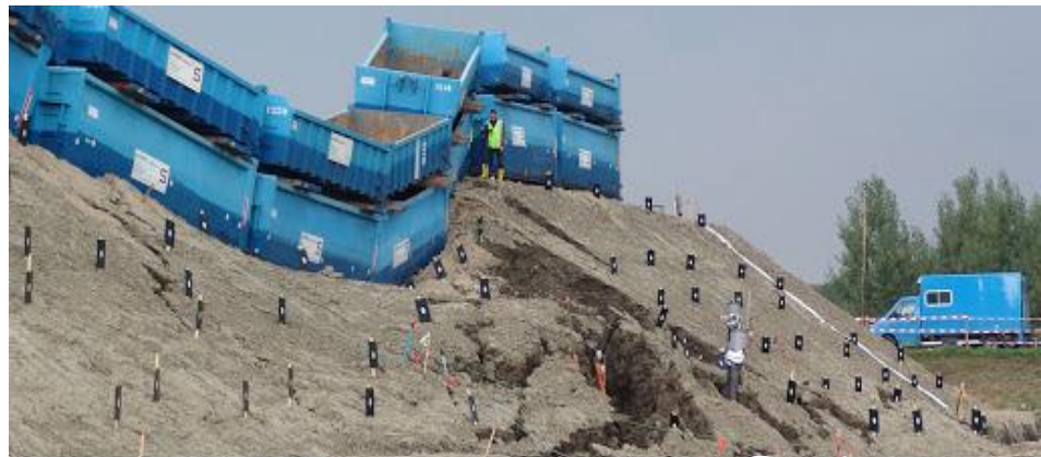
Dike breaches predictable thanks to sensor systems. The smart application of new monitoring techniques leads to significant cost savings and deferred investments for water authorities.
